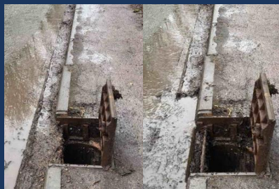
C1251 Whitchurch Side entry gully cleared
